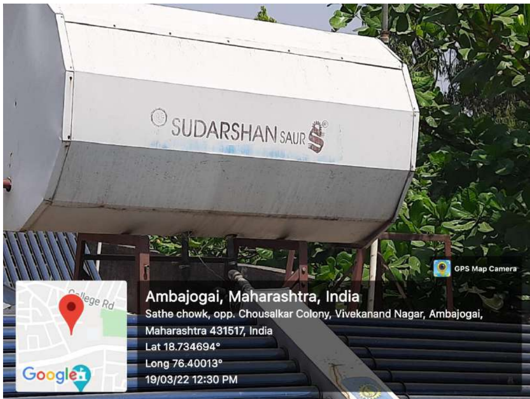
Solar system in Girls Hostel
