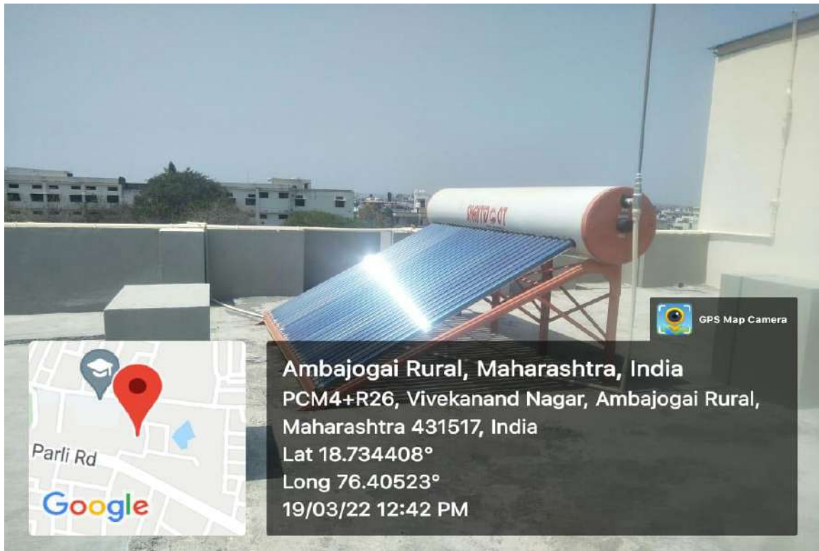
Solar System in Boys Hostel
