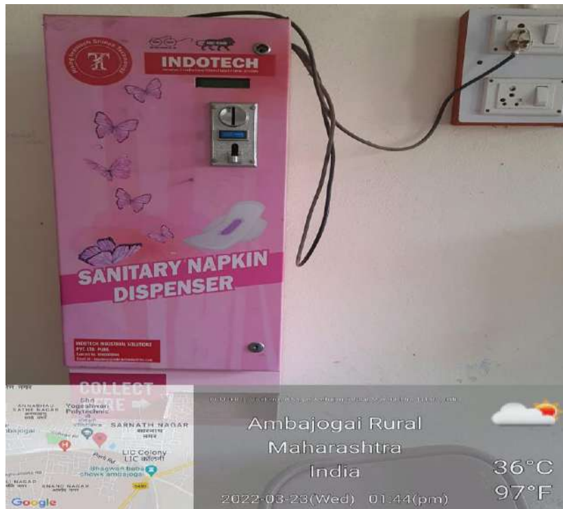
Sanitary Facility in Ladies Room
