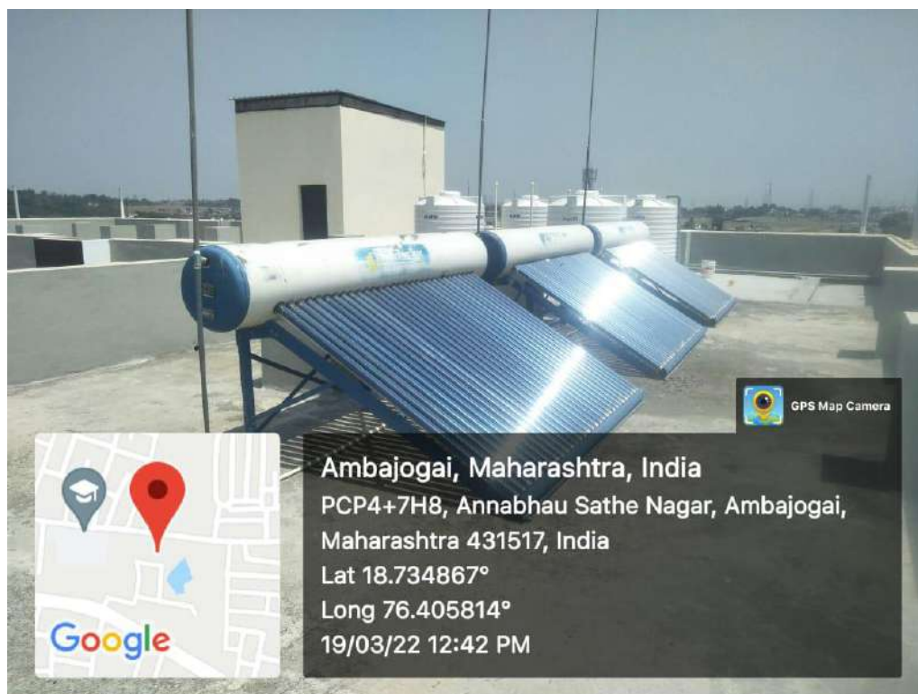
Solar system in Girls Hostel
