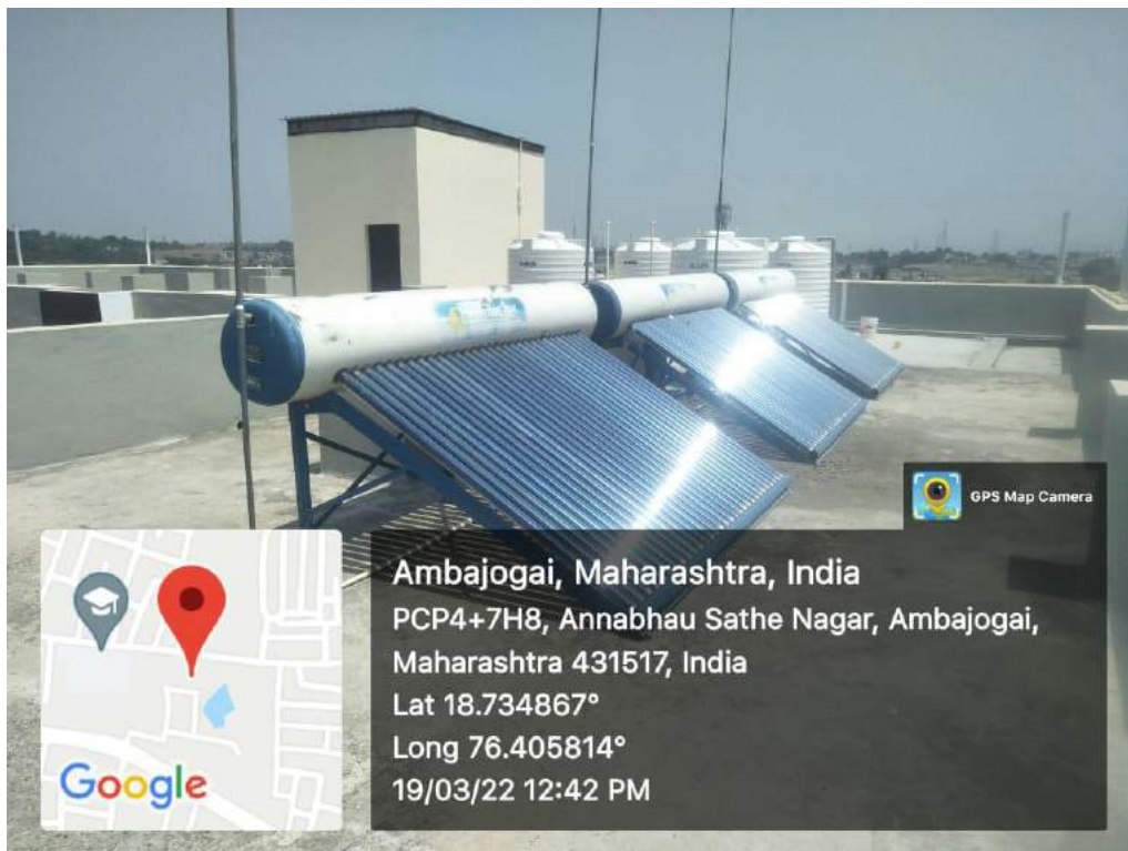
Solar system in Girls Hostel
