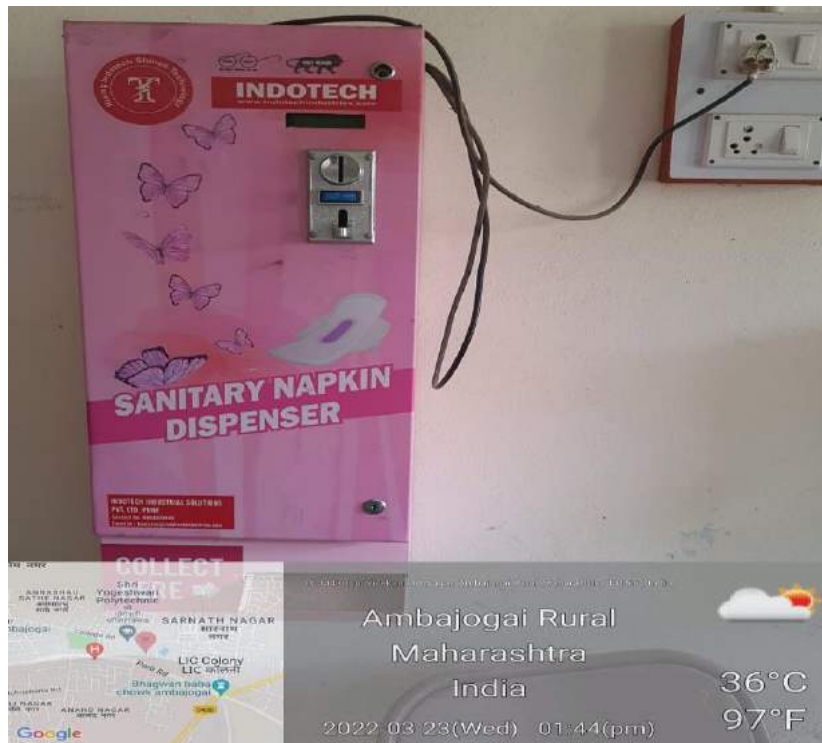
Sanitary Facility in Ladies Room
