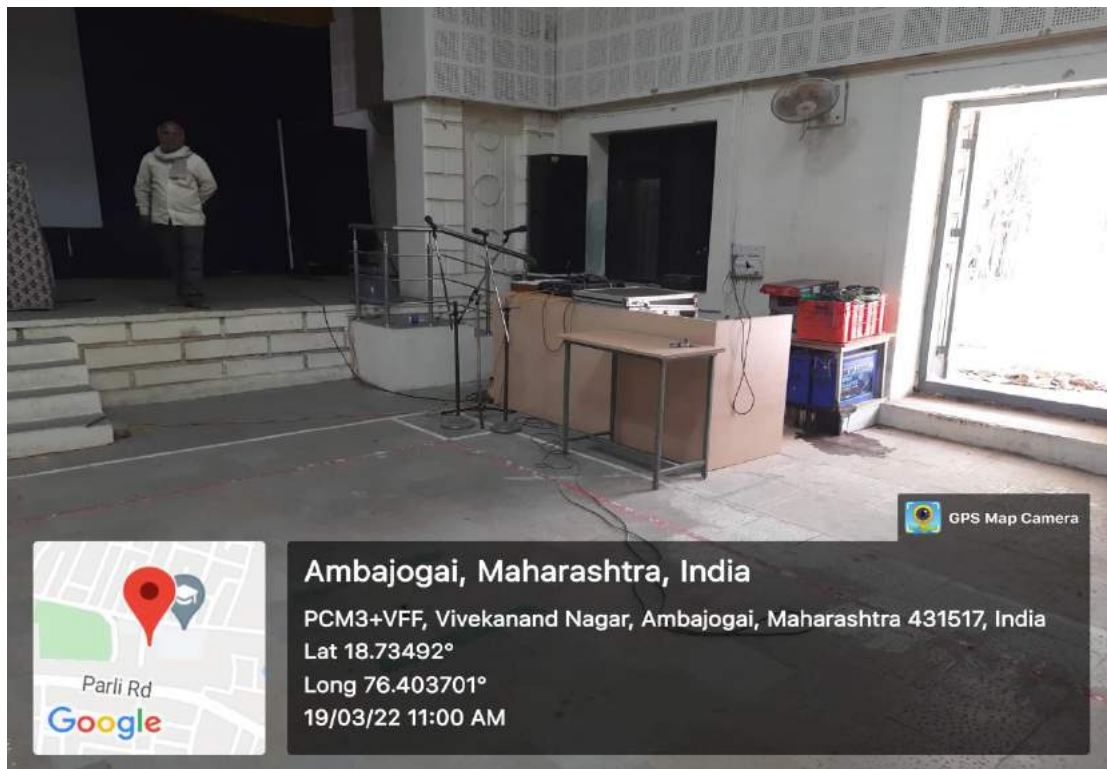
Mic and Control system of Auditorium
