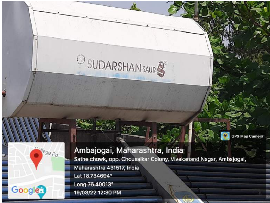
Solar system in Girls Hostel
